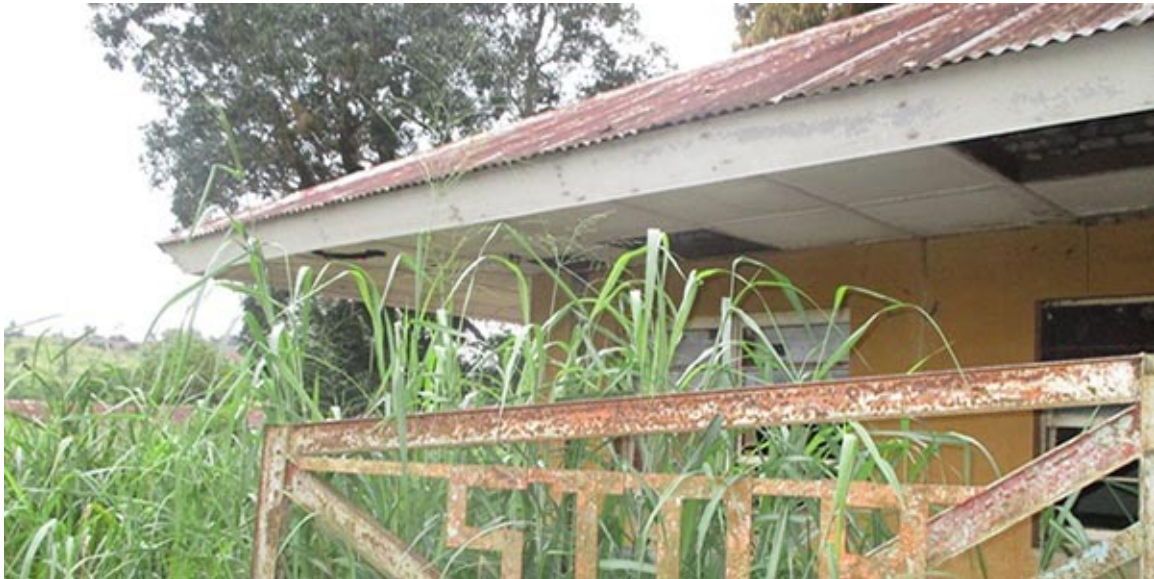
Ruines of Unilever's facilities in Lusanga, DRC. Ph: WRM.
